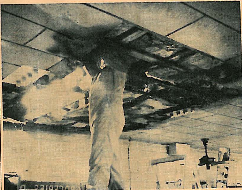
Workman starting to repair damage to ceiling and roof of Florence's Market caused by fire last Tuesday morning. Echo Photo.
