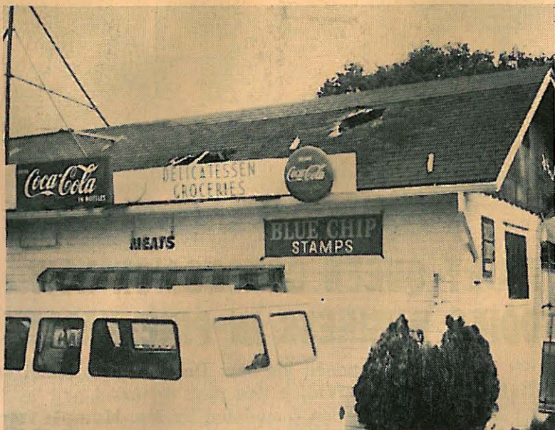
View of holes in roof of Florence's Market caused by fire. Echo Photo.
